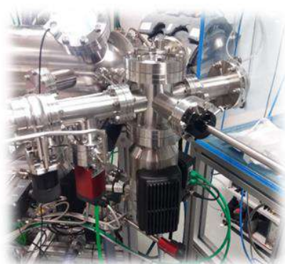
Customer installation example
